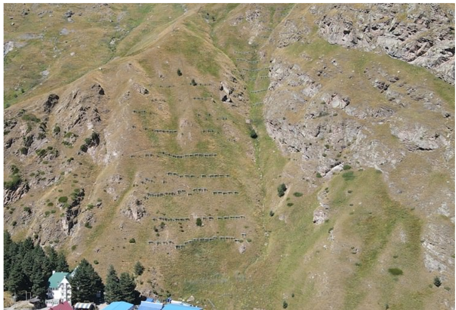
Figure 6. Snow retention structures on the southern slope of Mount Elbrus. Photo August 2022.
